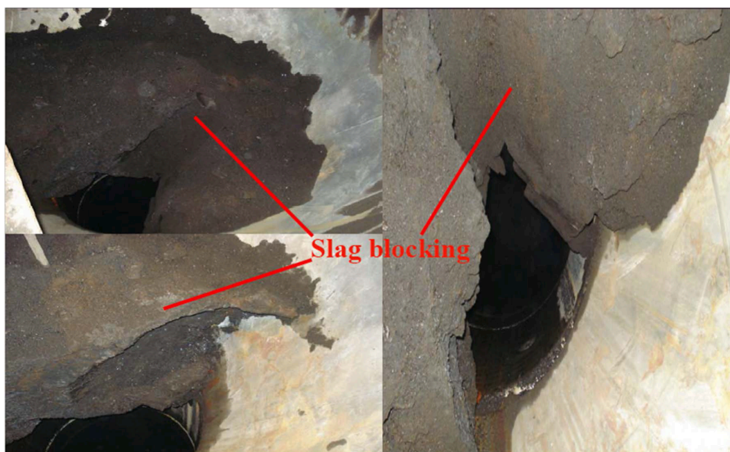
Fig. 1. The blocking of slag discharge system of Shell gasifier.
