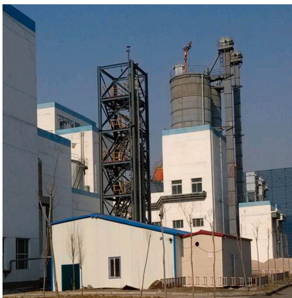
Fig. 9. Photo of 1000t/a CO 2 capture pilot plant in Changchun Thermal Power Plant.
