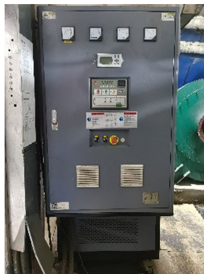
FIGURE 2 The photo of the working fluid circulation heater
